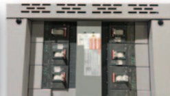
Feeder sections 45"-60" wide
