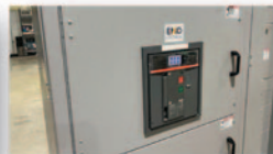
ABB engineering and innovation
