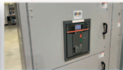
ABB engineering and innovation
