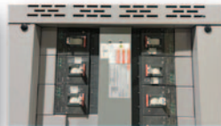
Feeder sections 45"-60" wide
