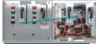
Siemens MCC Buckets
