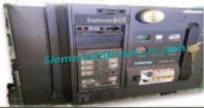
WL Low Voltage Breakers
