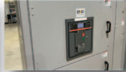
ABB engineering and innovation
