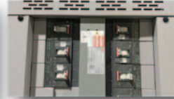
Feeder sections 45"-60" wide
