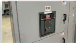
ABB engineering and innovation
