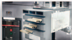
Switchboards covering the industry standard
