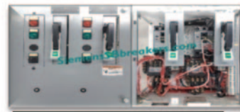
Siemens MCC Buckets
