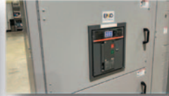
ABB engineering and innovation
