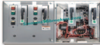
Siemens MCC Buckets
