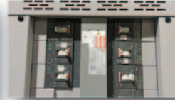
Feeder sections 45"-60" wide
